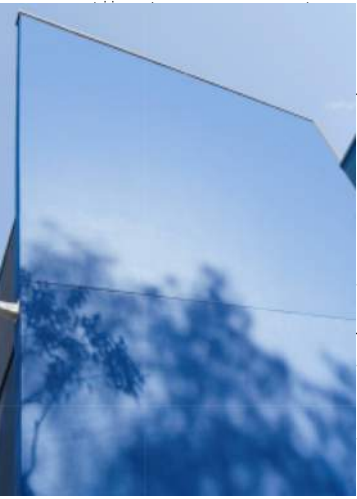
CON01 PRECAST CONCRETE PANELS
